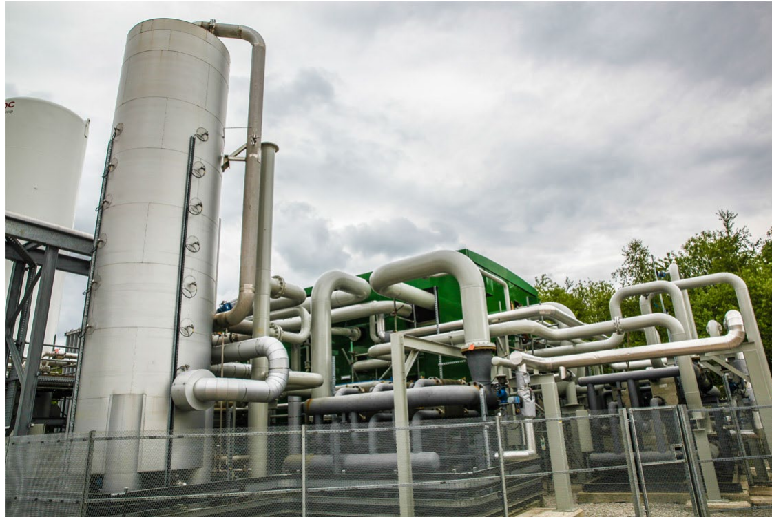
5-MW LAES demonstration plant, Manchester, UK
