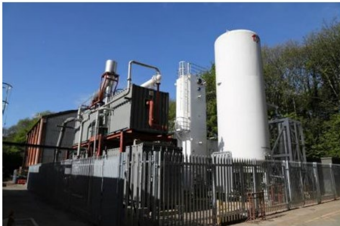
350-kW LAES pilot plant, Birmingham, UK
