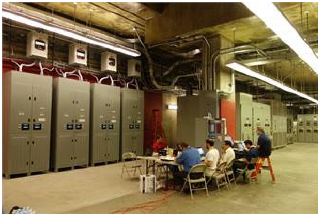
2-MW FES unit at metro substation, LA, USA
