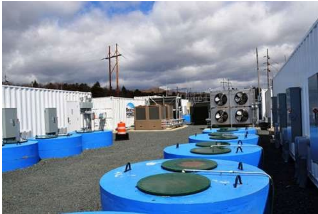
20-MW FES plant, Stephentown, NY, USA
